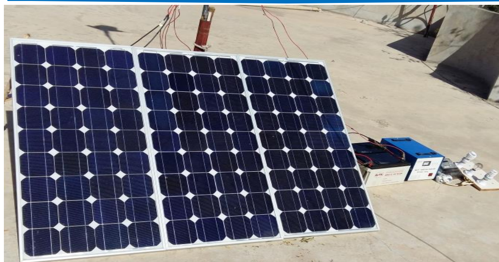
Figure 6 Energy Generation by three Solar panels of 80 W.
