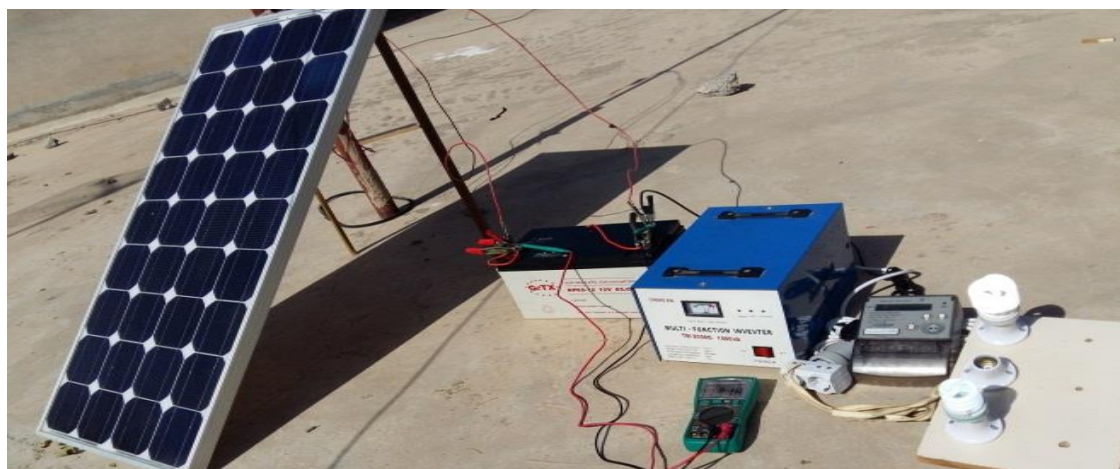
Figure 4 the photography of the one-panel solar panel system connections and components.
