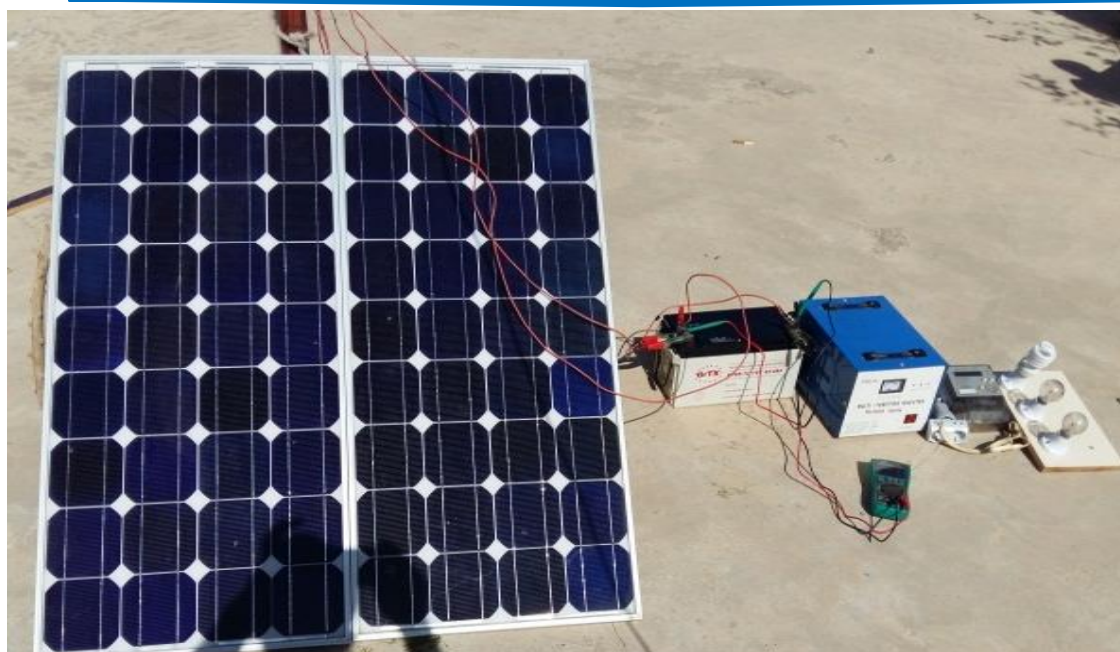
Figure 5 Energy generation by two solar panels of 80
